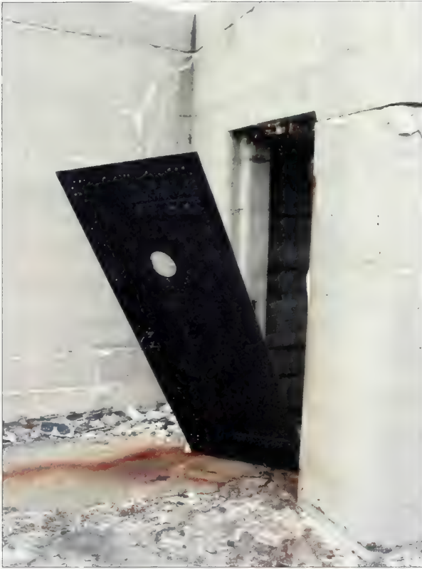
Figure 3.17. View of failing metal door, Nine Gun Battery. Several dozen doors and windows are missing or not properly mounted at the magazines, commander's stations, and other auxiliary rooms at Nine Gun Battery (Olmsted Center, January 2009).
